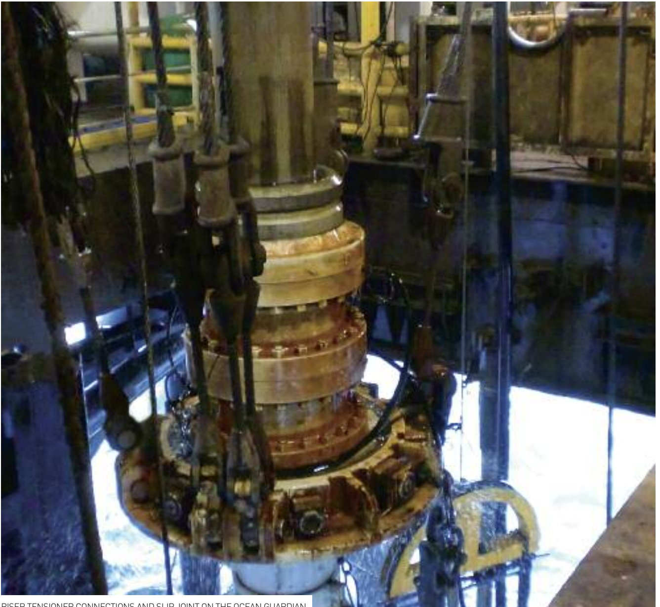
RISER TENSIONER CONNECTIONS AND SLIP JOINT ON THE OCEAN GUARDIAN
